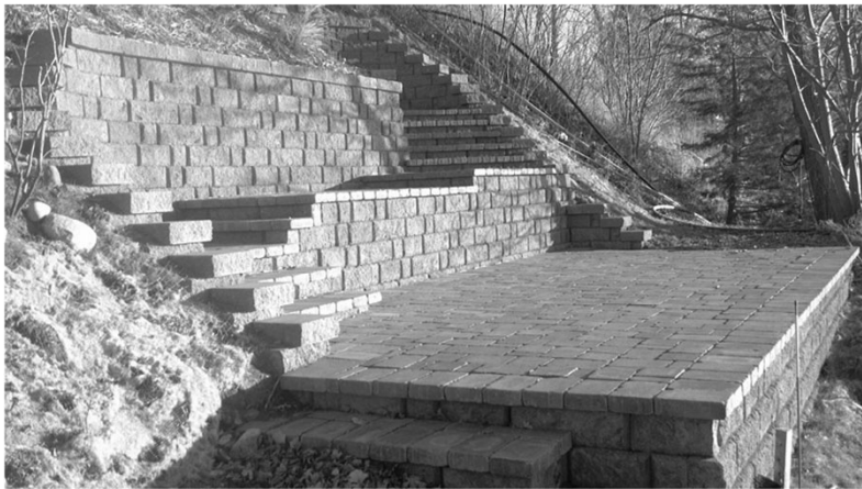
Guardrail missing or not installed (Patio)
