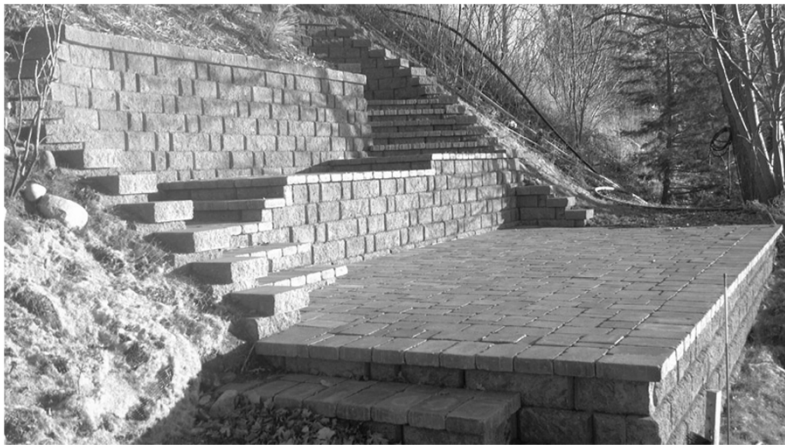
Guardrail missing or not installed (Patio)
